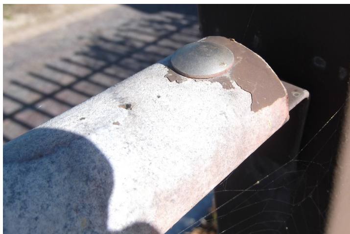
Corroded zincalume fence showing white zinc and aluminium corrosion product
