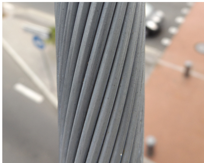
Galfan coated wire rope in a coastal environment
